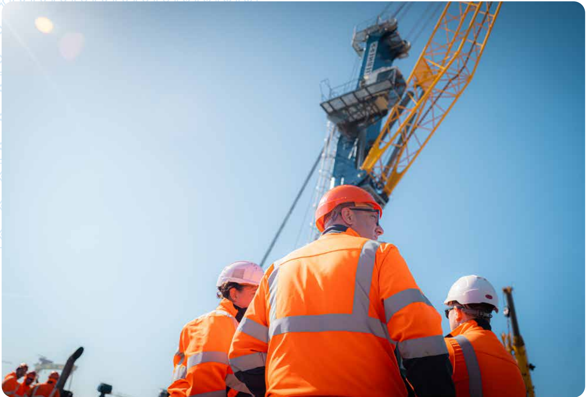
A new crane being installed in spring 2026, as part of our Horizon 1 crane upgrade plans.
